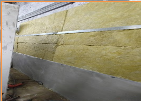
Industan Rubber, Mumbai ( AHU Room Accostic)
