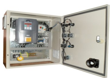
VFD Control Panel
